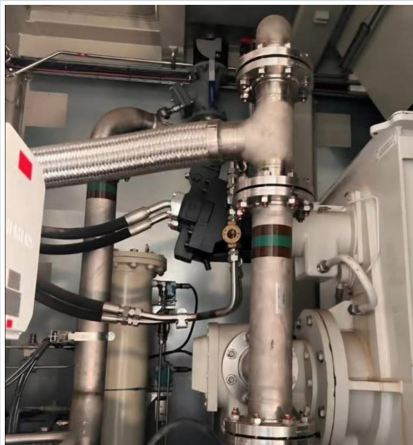
Package piping, flexible connection, and auxiliary interfaces
