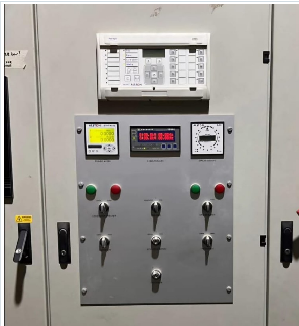
Generator protection, metering, and local control panel
