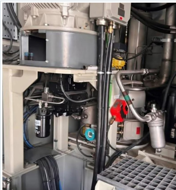
Auxiliary equipment, filtration, piping, and cable routing
