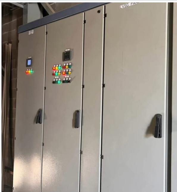
Low-voltage switchgear panel lineup
