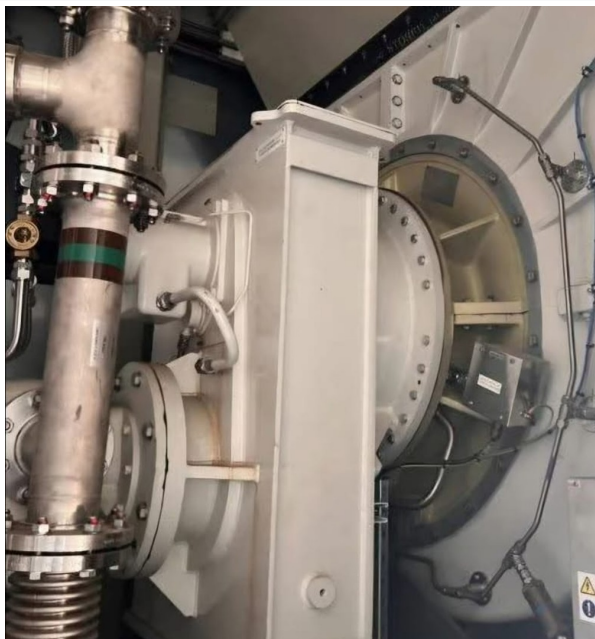
Package casing and large-bore auxiliary piping
